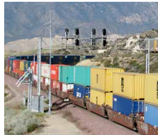
A positive train control radio tower stands next to a signal bridge on the BNSF main line at Cajon Pass. Carl Massart
